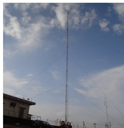
Fig. 2 – Detail of the mast and main station.
